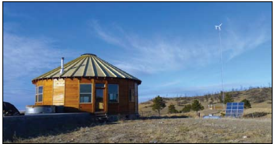
A yurt—economical in and of itself—powered with PVC panels and a wind turbine (right).
